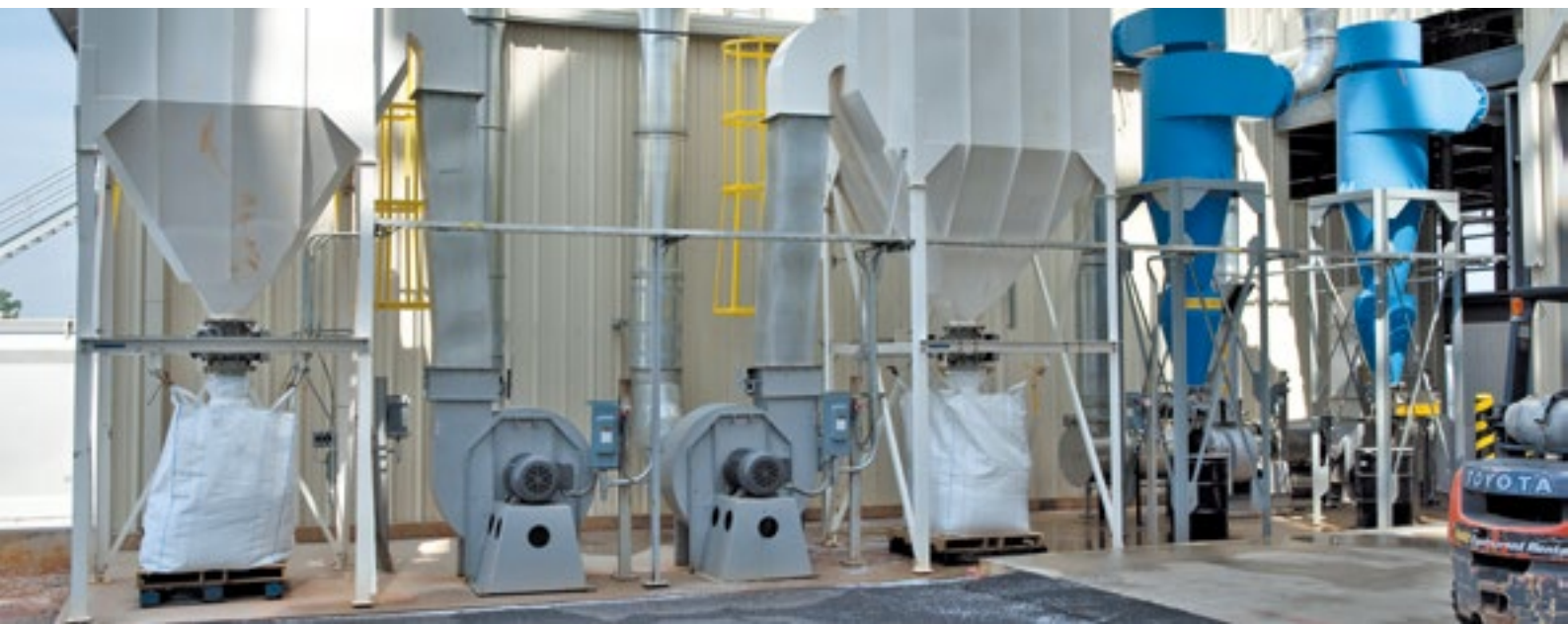
Fans, bag house and cyclones for a dedusting system
